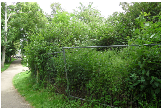
The section of Hiscock’s ‘Waterloo Bridge’ wall adjoining Druitt Gardens is overgrown and fenced off due to fears about its stability (photographed June 2016).
