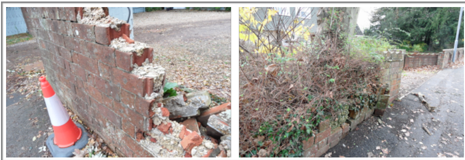
Photo 2: Left - Section showing the interlocking style of the bricks; Right - The damaged caused by tree roots in another section of the wall
