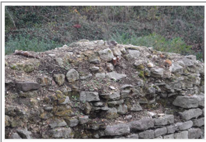
Photo 3: The walls clearly still remain in a precarious state
